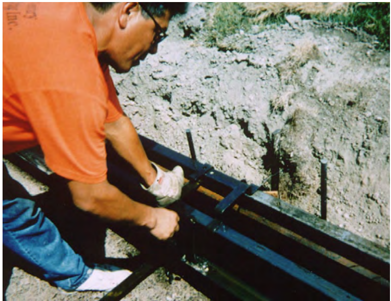
Place the Top Spreader over the forms to secure the Curb Face Form.
